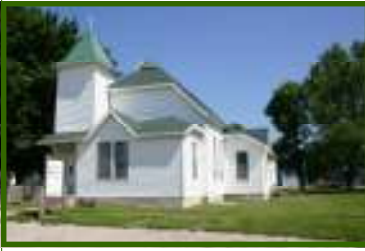
Blue Mound UMC, note the new roof with all its slopes and gables.
